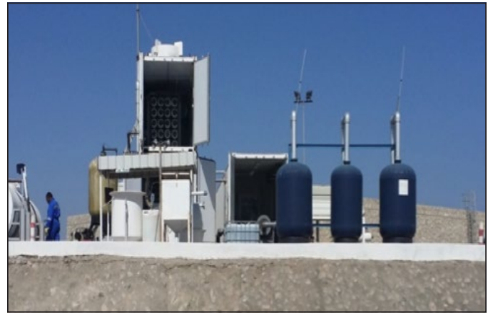
An overview of Al-Kuwiama RO desalination plant
