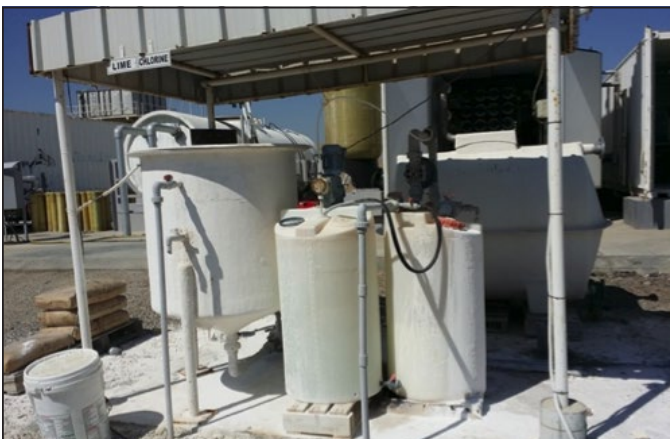
Treatment point for pH and chlorination
