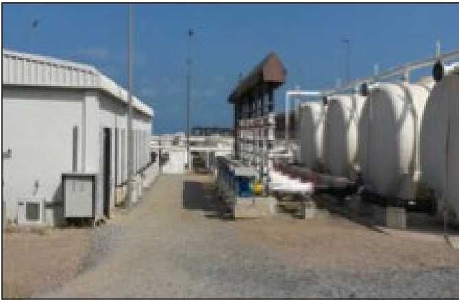
Al Ghubrah seawater reverse osmosis desalination plant
